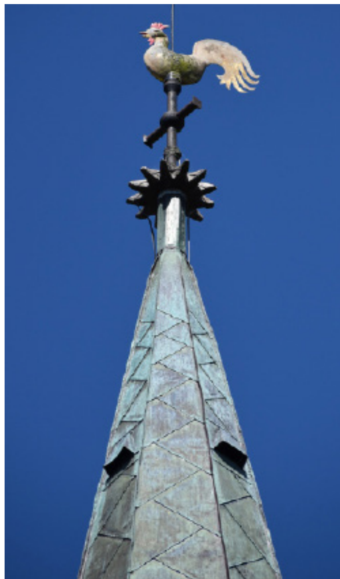
Although lead is the most common metal roofing material used historically, copper was widely used for decorative effect, as here on the steeple of St Mary's, West Harptree. (Photo: Jonathan Taylor)
