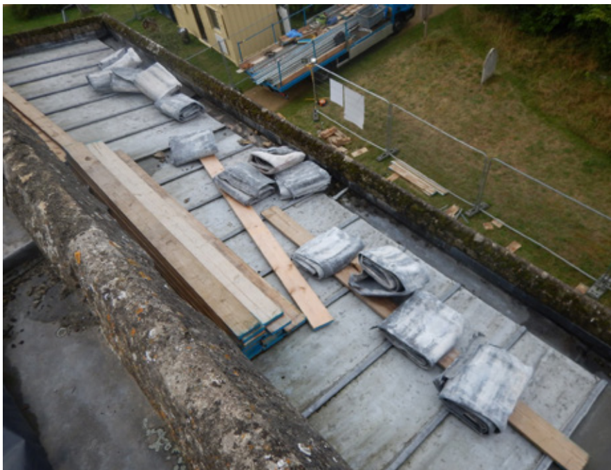
St Mary the Virgin, Kirtlington, Oxfordshire, with neatly rolled up sheets of lead left by in a hurry by the burglars (Photo: Angus Brown)
